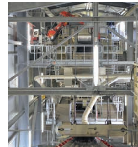
Vorbrechanlage, Rohgips, 400t/h, HAVER F-CLASS, Plattenband, Backenbrecher
