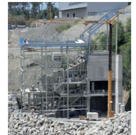
MASTER Vorbrechanlage, Kalkstein, 600t/h, HAVER F-CLASS, HAVER Schubwagen, Prallbrecher
